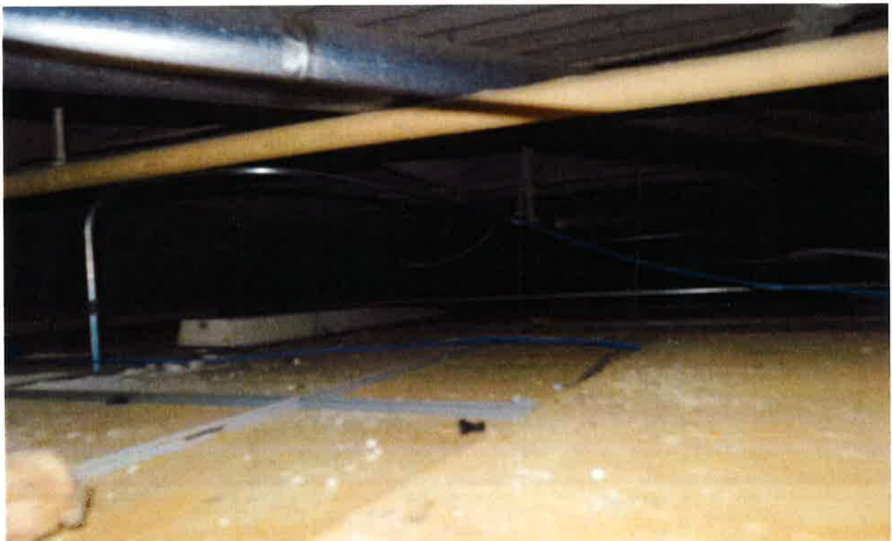
ACM debris on top of ceiling tile on 10 th floor. This space is also the return air plenum.
