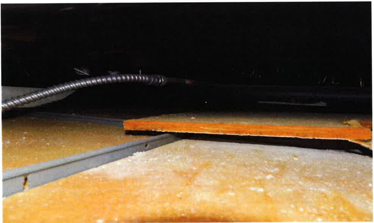
ACM fireproofing debris on ceiling tile in the return air plenum of the 2 nd floor
