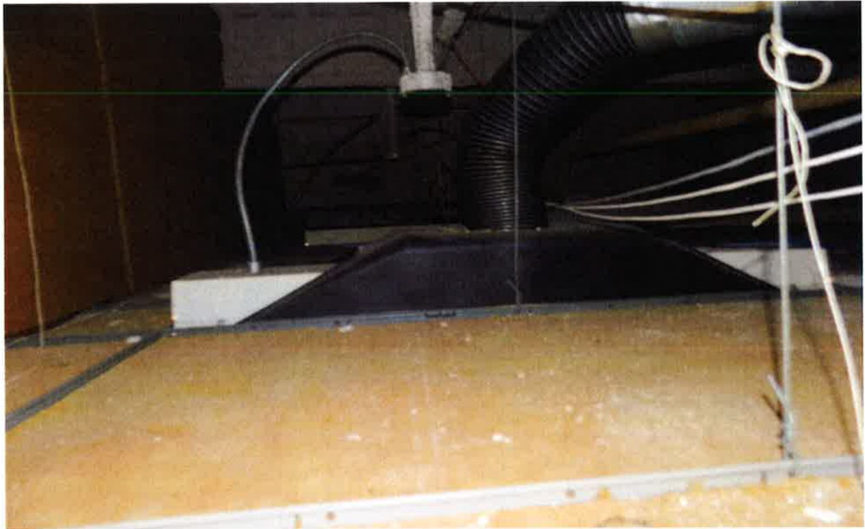
ACM fireproofing debris on top of ceiling tile on 10 th floor. This space is also the return air plenum.
