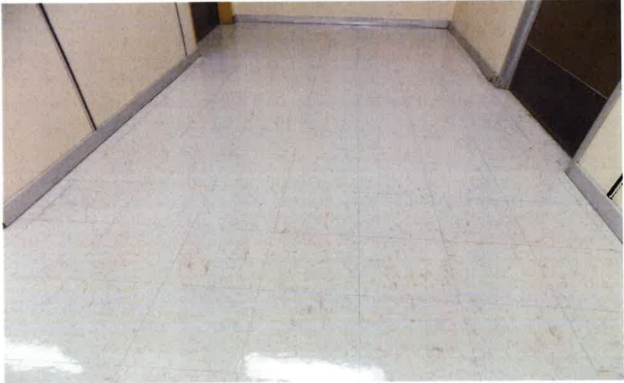
ACM 9 X 9 floor tile and mastic prevalent through out building
