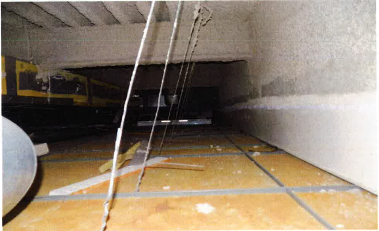
ACM fireproofing debris on ceiling tile in the return air plenum of the 2 nd floor
